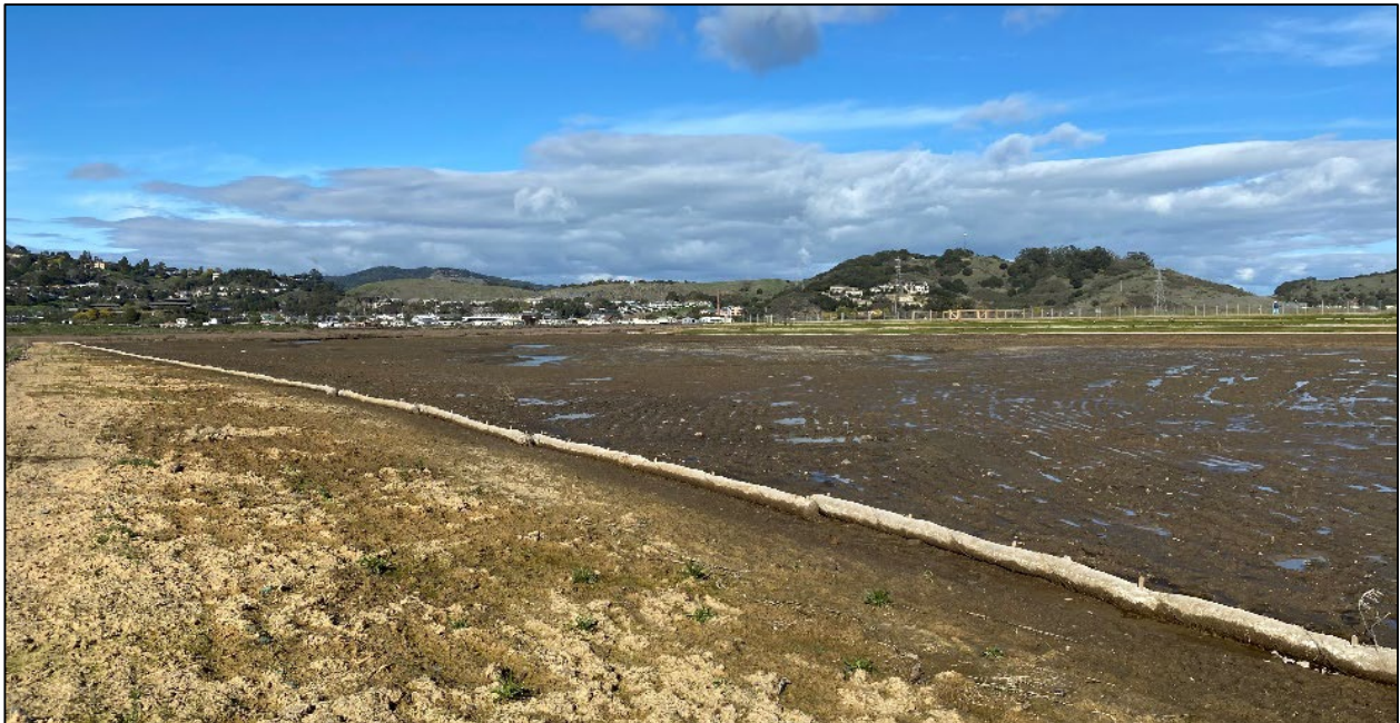
Post-construction Photo Point 8: View of new transition zone and tidal marsh, facing northeast. Photo taken February 12, 2021.
