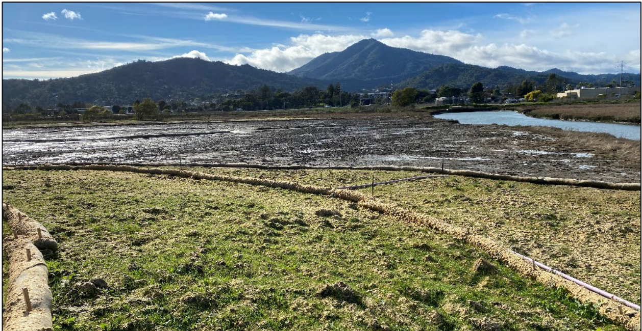
Post-construction Photo Point 1: View of new transition zone and tidal marsh, facing west. Photo taken February 12, 2021.
